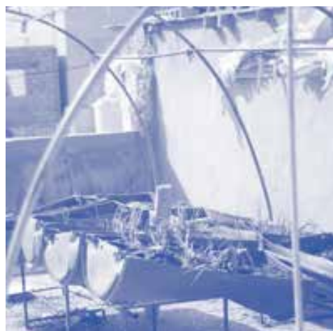
fig. 76: Broken greenhouse due to wind (own photograph)
